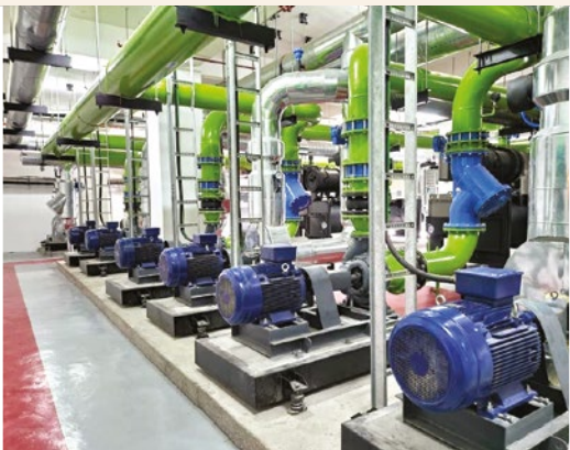
Chiller Water Pump System
