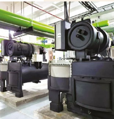
Chiller Plant Units
